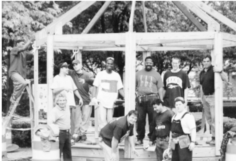
TEAM EFFORT... Students from the Union County Vocational-Technical Schools in Scotch Plains, pictured last spring, construct the Victorian-style gazebo on the Village Green as a class project. Township officials and downtown merchants hope the new landmark, along with distinctive benches, banners and signs, will enhance the ambiance of the business district.
