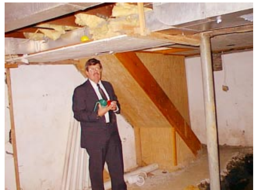
STILL NO SATISFACTION... Westfield resident Burton Michaels stands in the basement of his Everson Place house three years after a heating oil tank burst when it was apparently overfilled during a routine delivery of oil. A hole in the ground filled with water, sewage and traces of oil sit where the former finished TV room existed.
